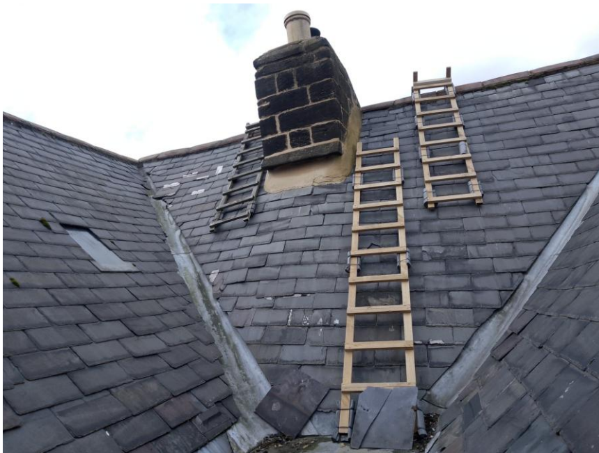
Figure 2: Photograph showing some of the PRFs around the roof tiles.
